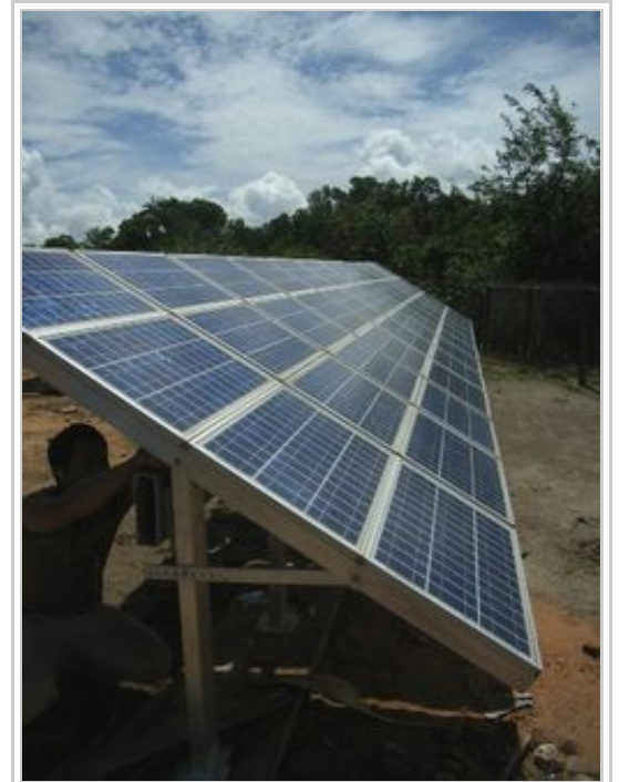
Figure 1. Solar PV array
